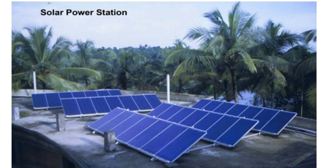
Section of the solar power plant in Mithradham
